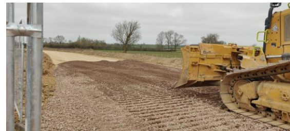
Images showing the development of our internal access road in our Twyford to Greatworth section
